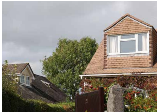
Figure 57: - Two styles of gable dormer, a pitched dormer roof is a more robust detail.
