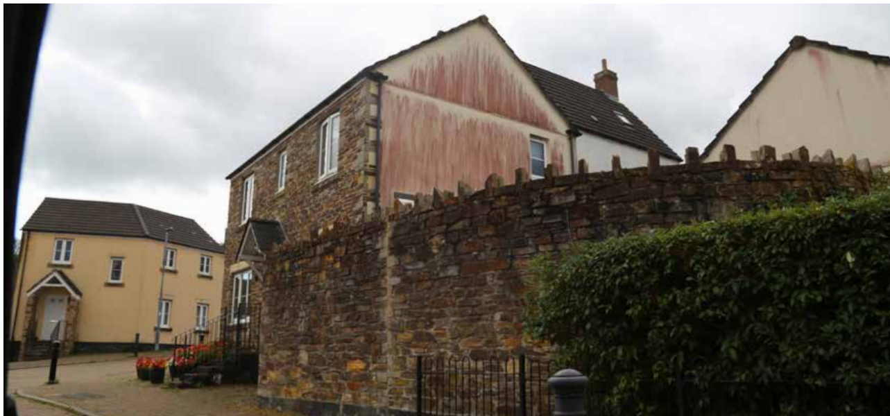
Figure 20: - 21st century example materials. Significant red staining shown on rendered facade.
